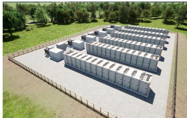
Battery Storage Compound
