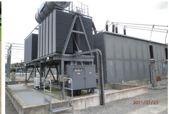
400 kV Power Transformer
